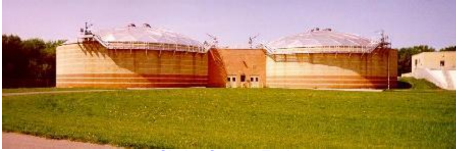
Sludge Storage Tanks
